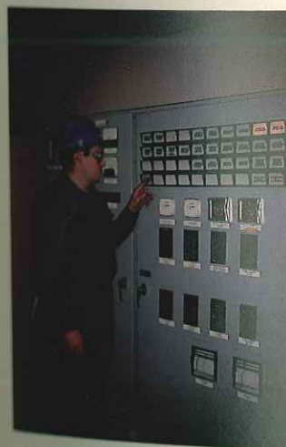
A mill instrumentation control panel with programmable logic controllers automatically monitors and adjusts milling operations.
