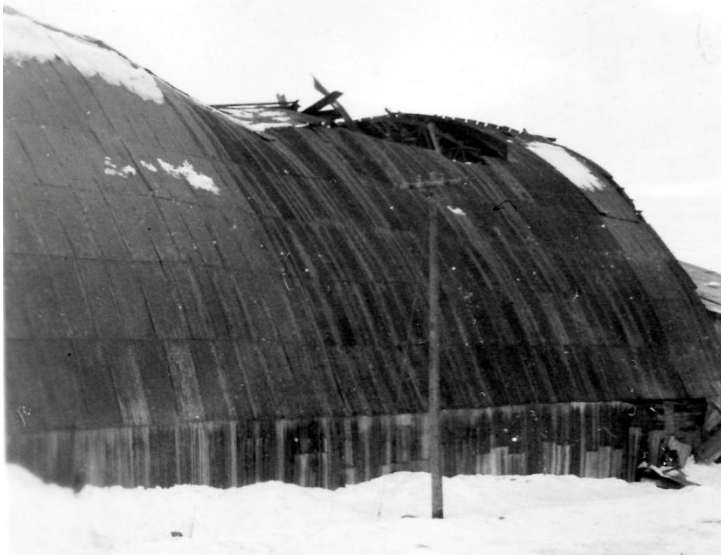
The Cobalt Arena Roof collapses on Christmas Day in 1940.
